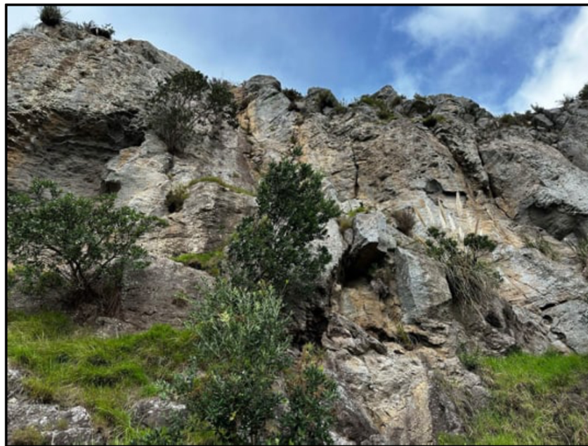
Figure 9: Susceptible joints and blocks identified on bluff outcrop above Te Ara Oruahine track, date taken 02/05/25.
