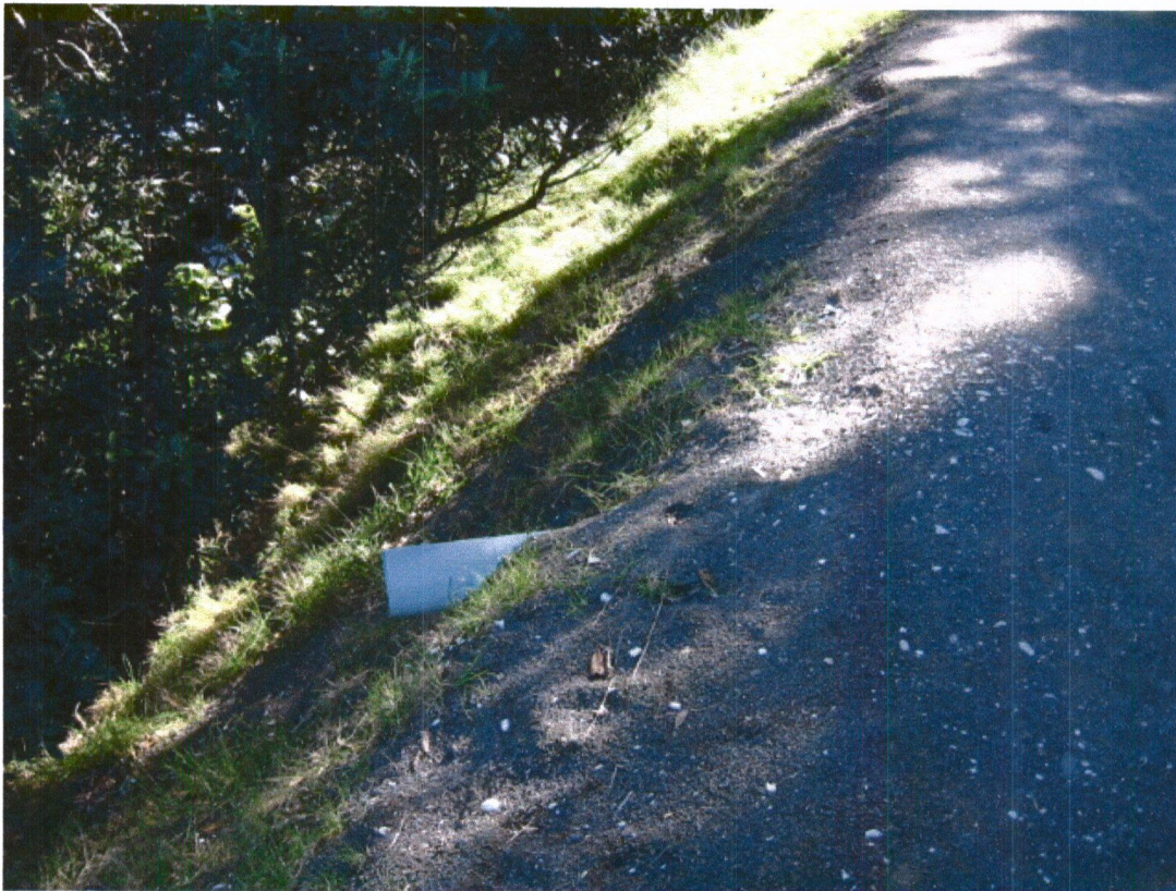
Projecting culvert pipe outlets encourage slope erosion Note the surplus track surfacing aggregate that has migrated off the track
