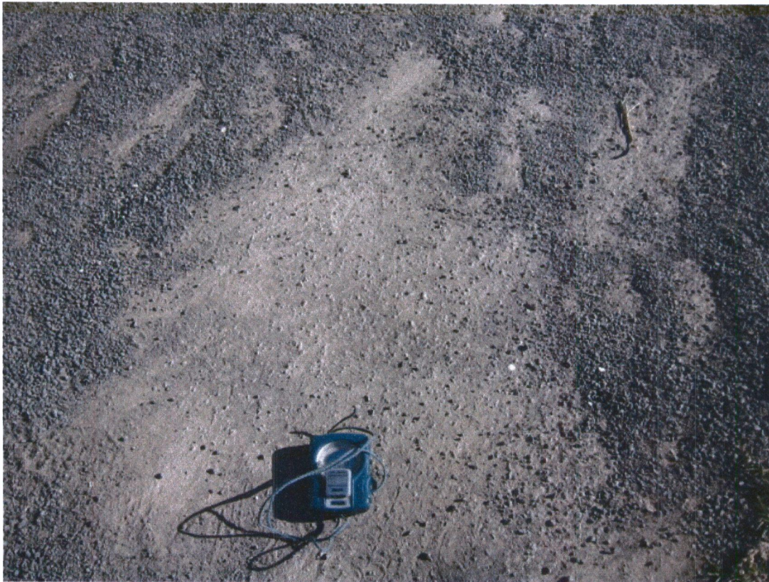
A suitable bound walking surface below the loose gravel Sweeping the existing track is recommended
