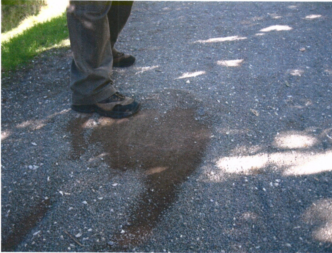
Loose aggregate on track surface represents a slipping hazard A "well graded" aggregate would provide a better bound surface
