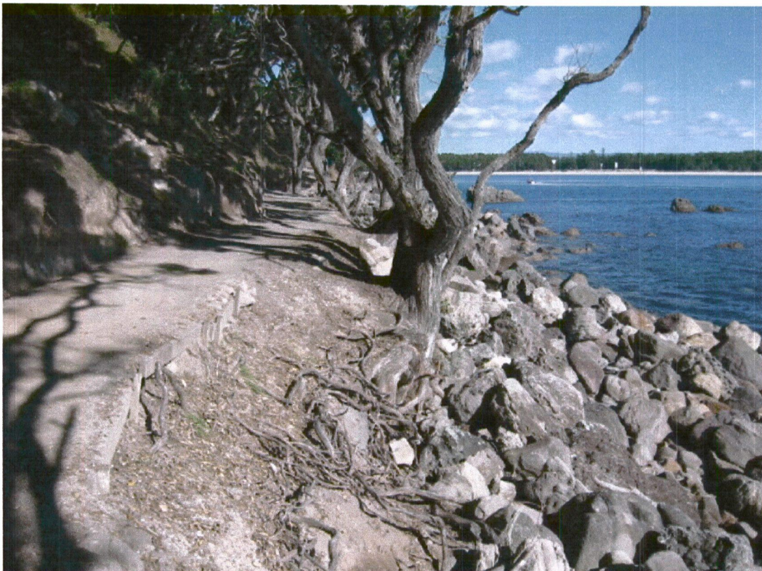
Coastal erosion and track undercutting from wave attack Armouring of the high tide line with local rock recommended
