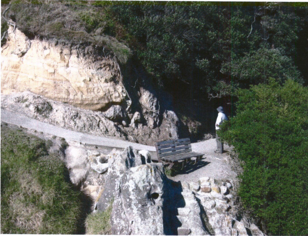
Short sections of track with 25% grade represent a slipping hazard Grade could be reduced by filling bottom of steeper sections
