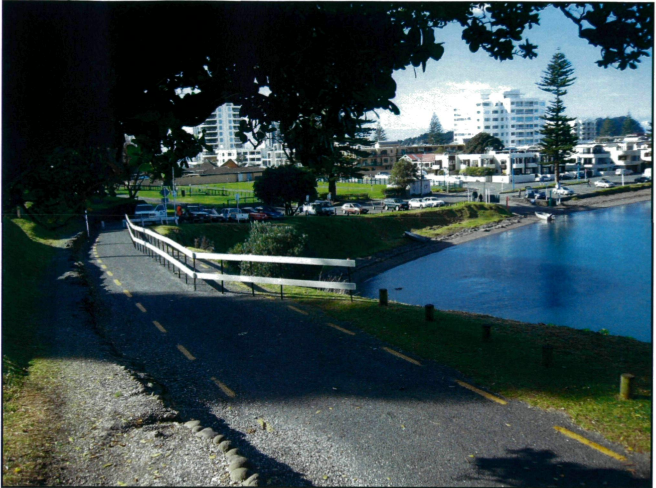
Figure 1 View toward boat launching area at Pilot Bay - Road slip defined by White fenced barrier
