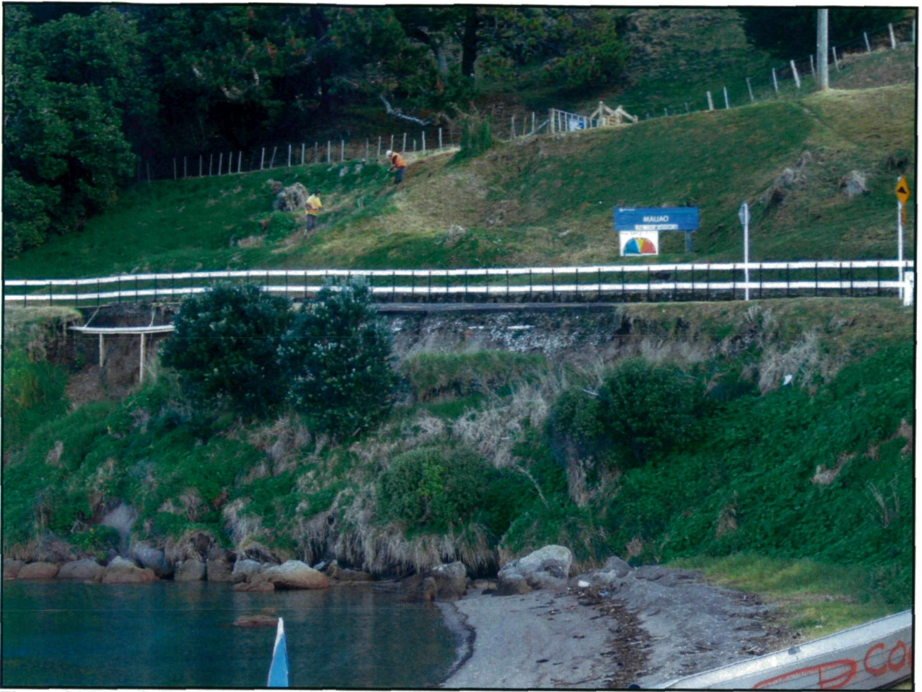
Figure 2 View of slippage from boat launching ramp at Pilot Bay
