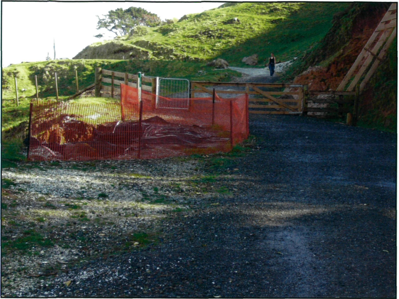
Figure 5 – 4W drive track and upper edge of the slip is defined by the temporary fencing.
