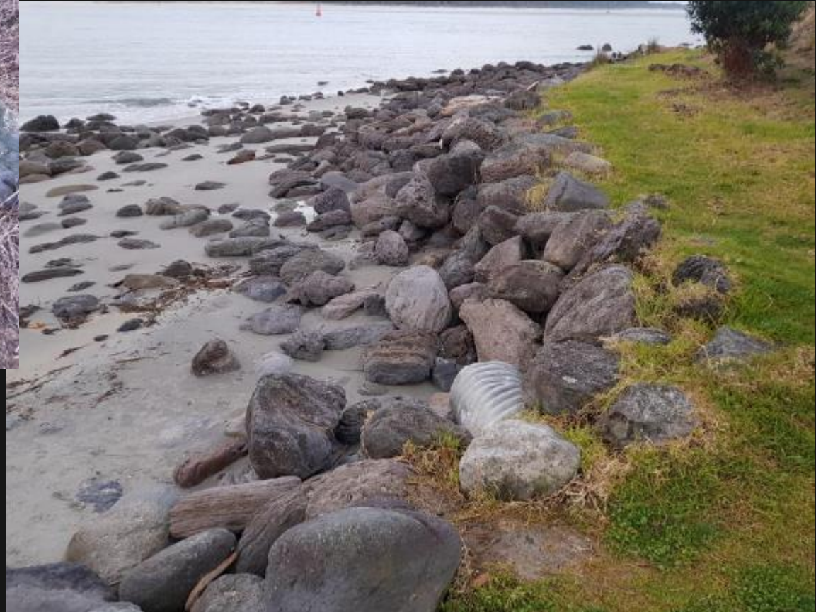
Current Storm-water outlet
