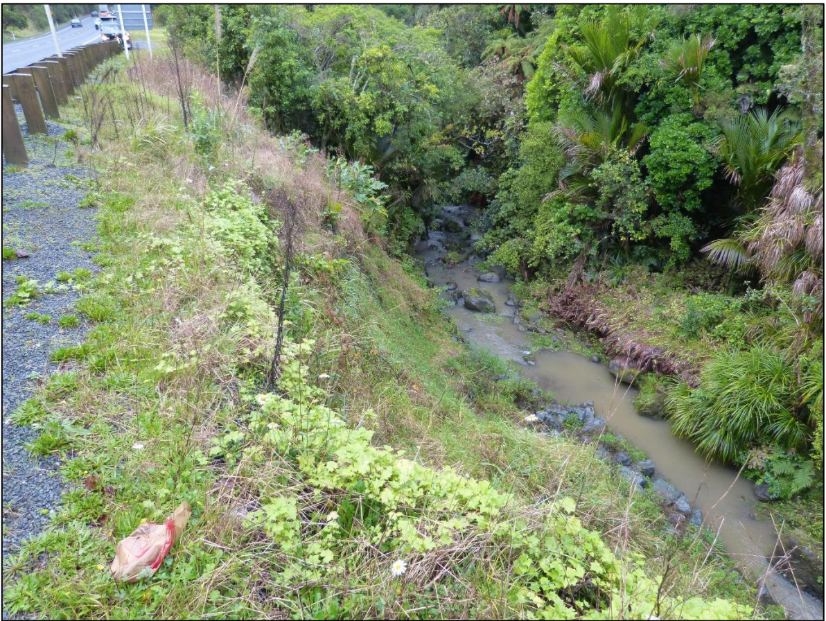
“Before and After” Showing natural revegetation of an Soilnail and Duramat repair
