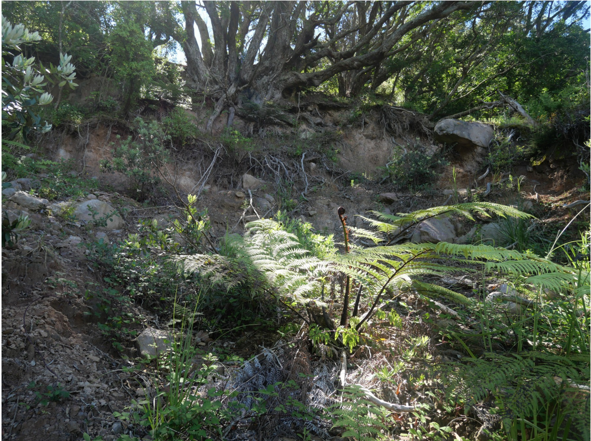
Photo 8. Active slip slope above the Goat track.
