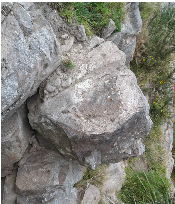
Photo 5 and 6. Loose rock identified on the bluffs above the Oruahine track.
