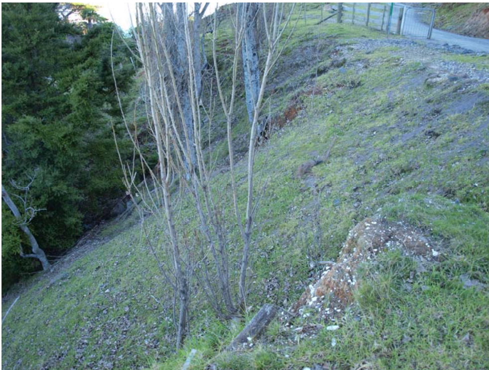
Photograph 10; Good remedial repair to a dropout below the lower 4WD track.
