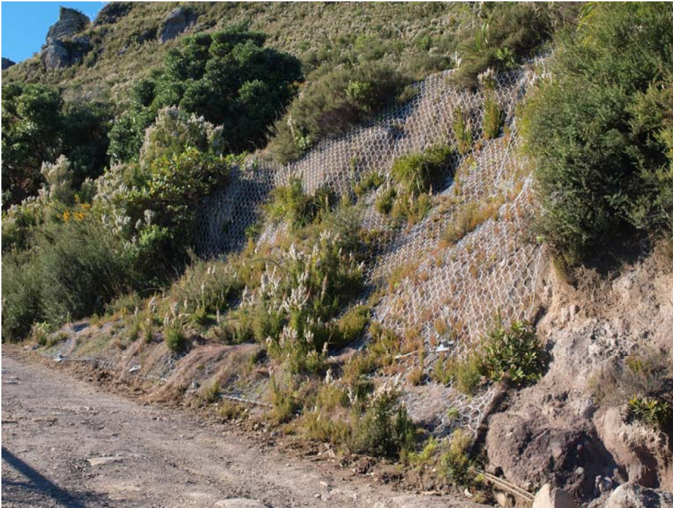
Photograph 6; The small patch of soil nails and mesh installed in 2005 to stabilise the 4WD track hairpin; performing well.
