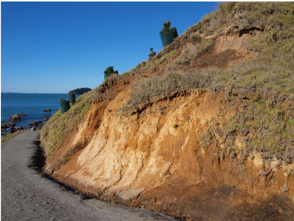
Photograph 9; Another slip scar above the base track.
