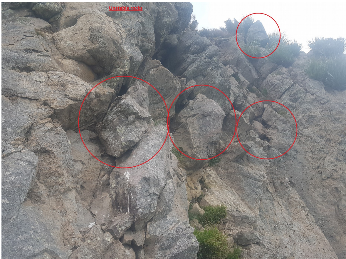
Photo 3. Loose rock above the Oruahine track.
