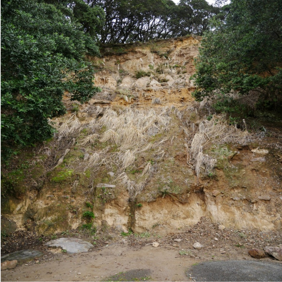
Photo 6; Eroding face above base track
