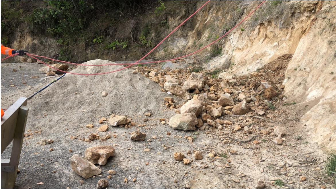
Photo 16; Rock removed from scoured slope face above the Western Base Track.
