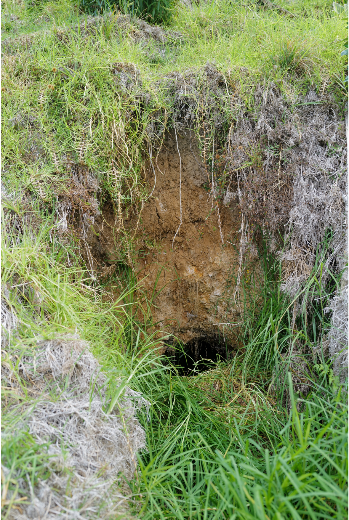
Photo 10; 2m deep 'sinkhole' / void collapse
