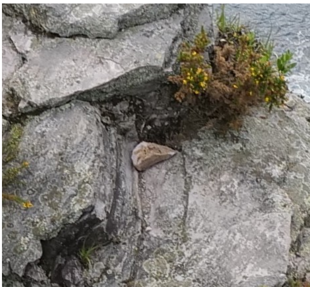
Photo 4; Fresh rock on top of column – detail in centre of photo 3, above.
