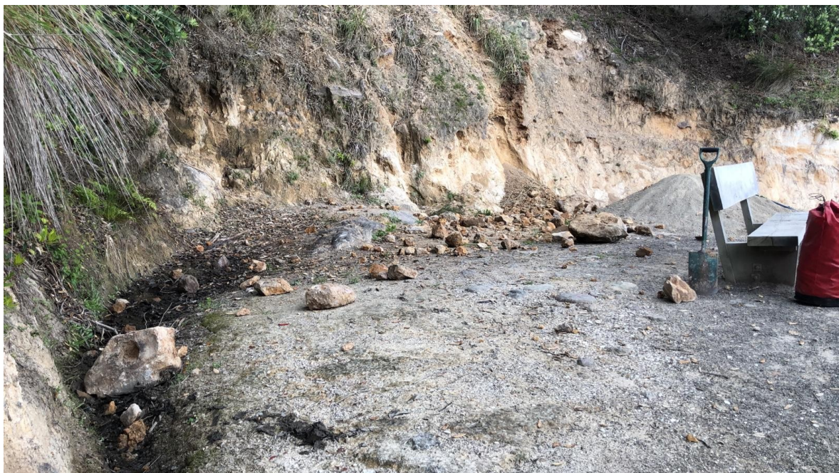
Photo 17. Rock removed from scoured slope face above the Western Base Track.
