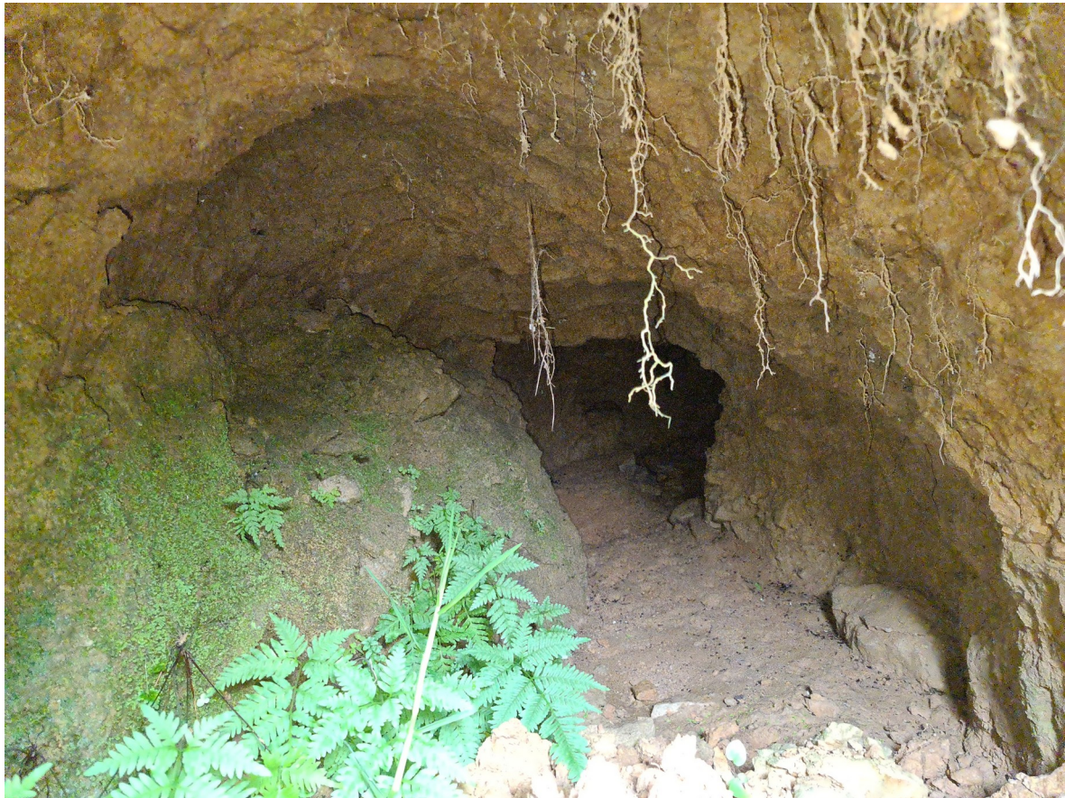
Photo 11; 'Tunnel' into slope from base of collapse hole.
