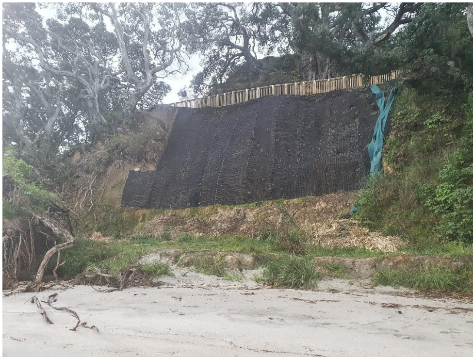
Looking towards the slip from the tidal platform. Photograph 18 (top) was taken during the first inspection on 02/06/20. Photograph 19 (bottom) was taken on 27/08/20.
