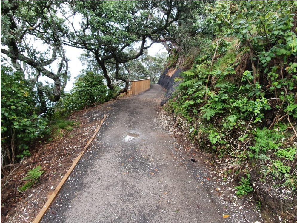
Photograph 1 - At the start of the track looking west - minor ponding on the track.
