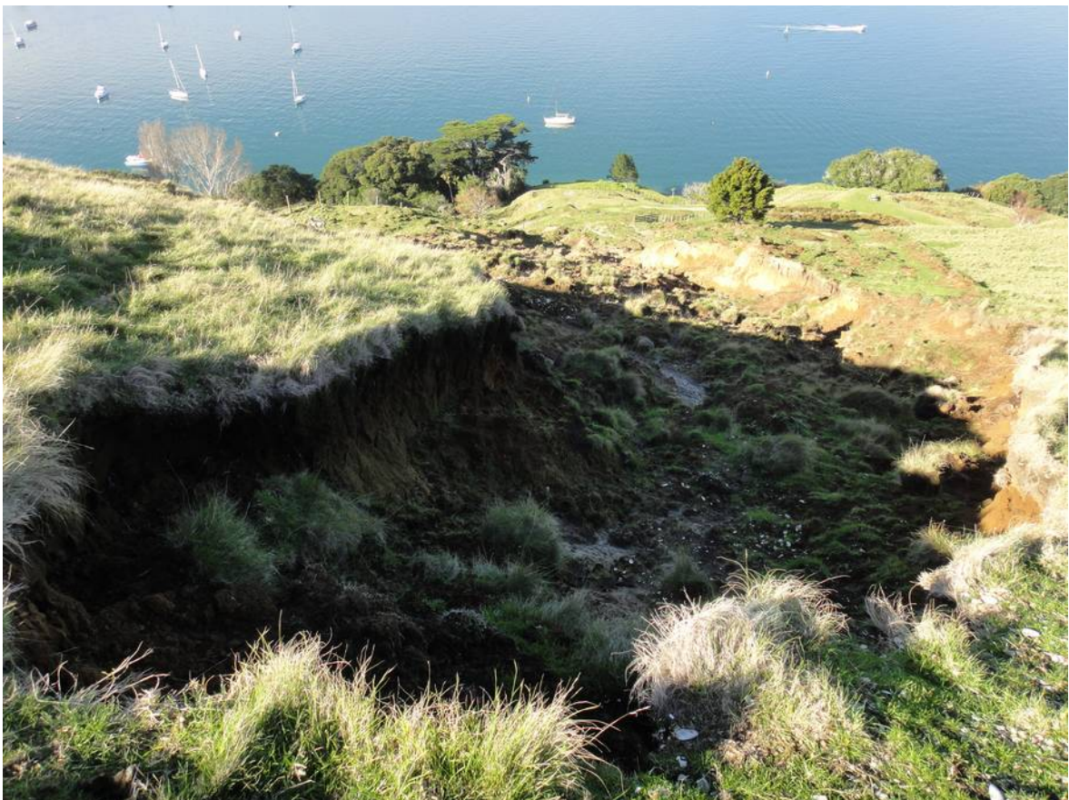
Photo 2; Slip reactivated on southern slope.
