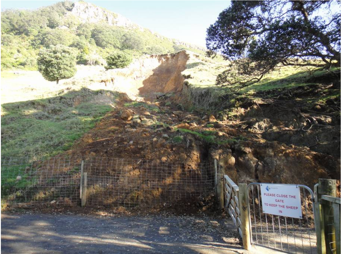
Photo 1; Slip adjacent base track immediately N of campground.
