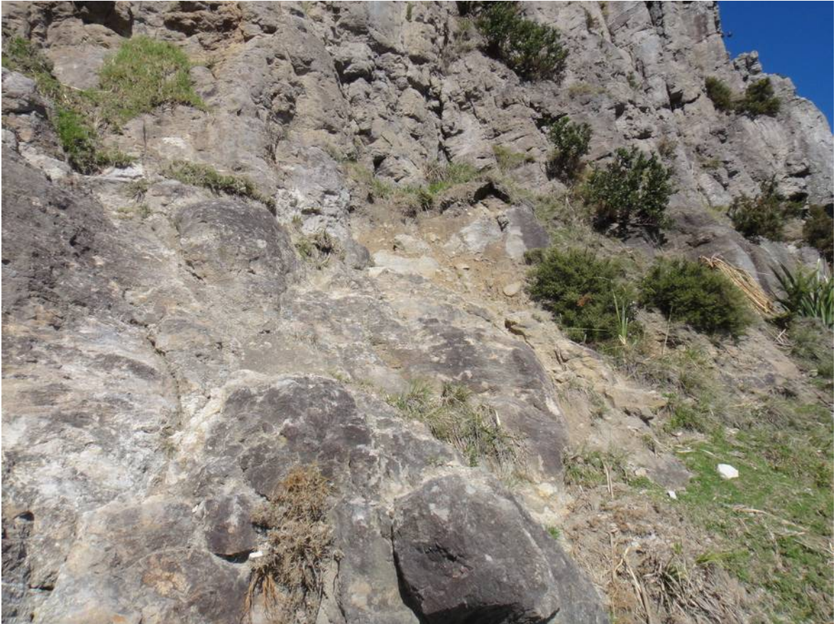
Photo 9; Small slip/rockfall source above Oruahine track.
