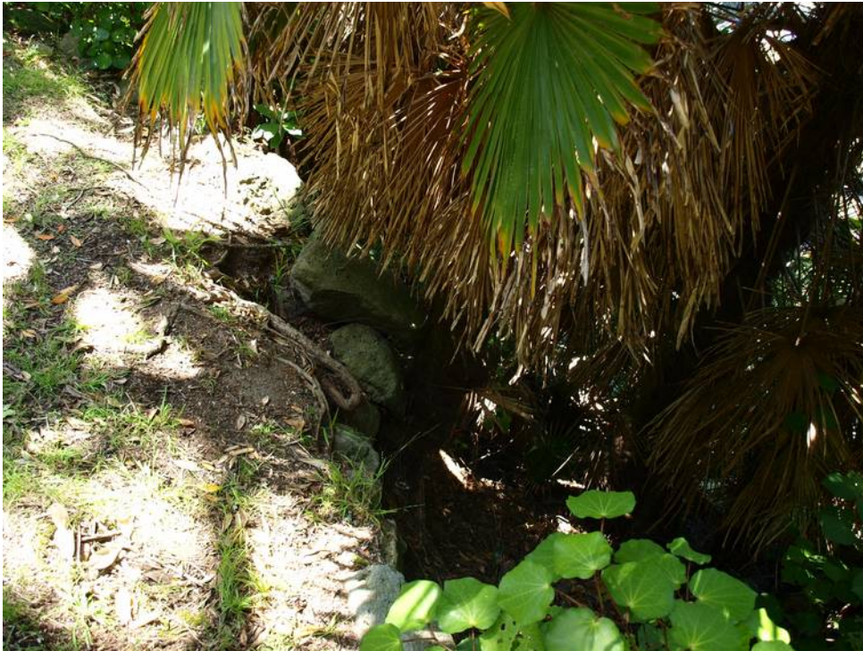
Photograph #9. Failure of retaining wall at top of cut slope behind camp site.
