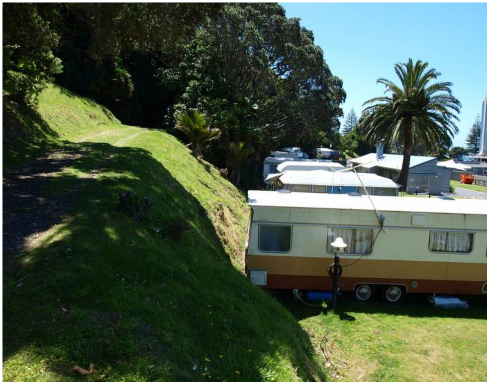
Photograph #10. The cut slope. Photograph #8 taken just behind the palm.
