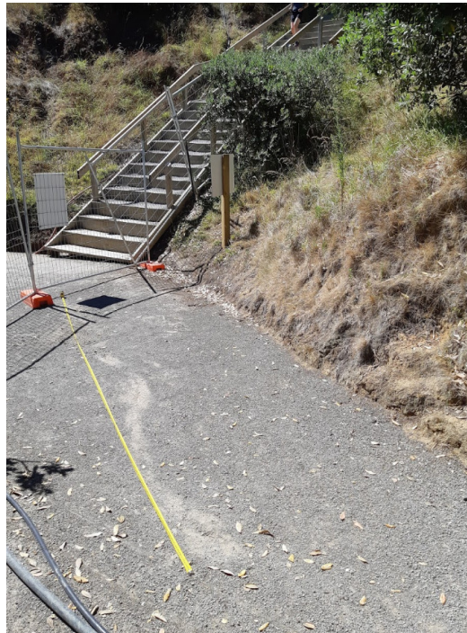
Photograph 2 - View of crack looking west
