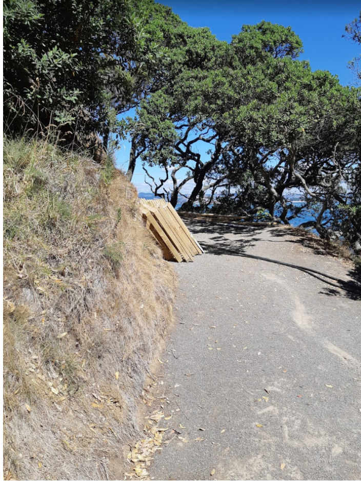
Photograph 1 - View of crack looking to the east
