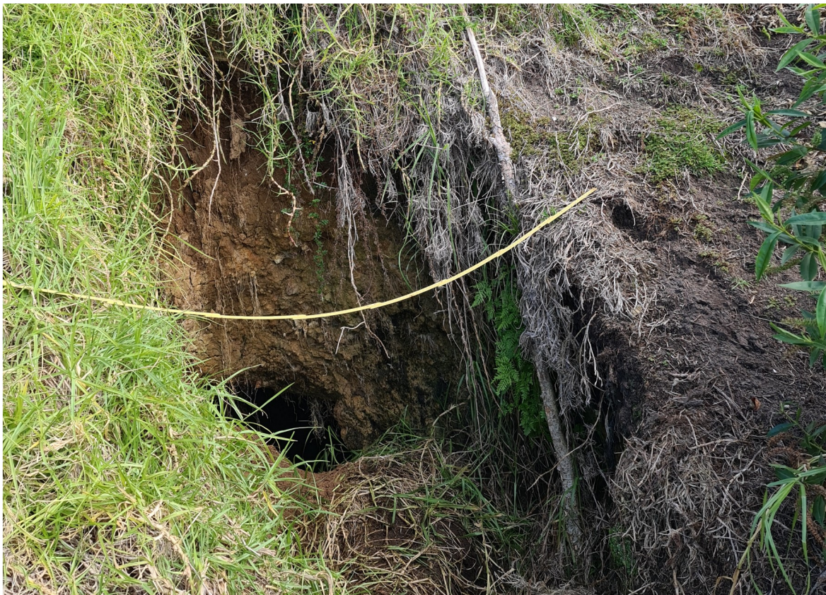
Photo 2; The sinkhole at the surface (2m scale).
