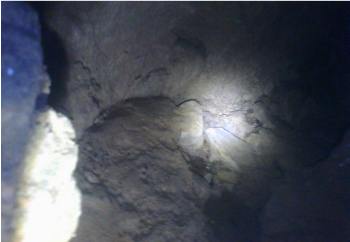
Photo 5; The tunnel continues to the right. Furthest view in photo is around 5m from the entrance. The diameter of the tunnel here is around 0.5m.
