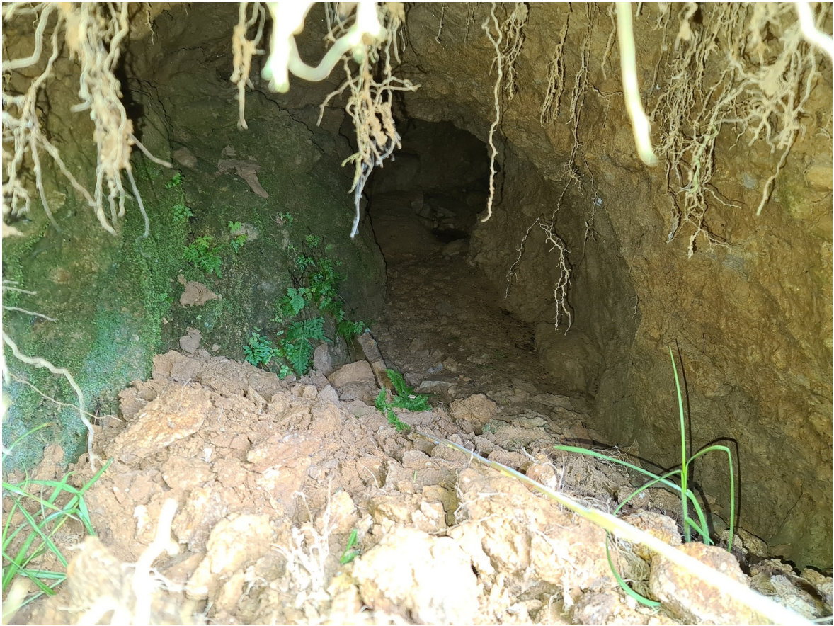
Photo 3; The sinkhole entrance.
