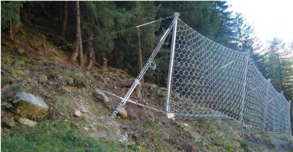
Figure 4: Flexible rockfall barrier (Source MBIE)
