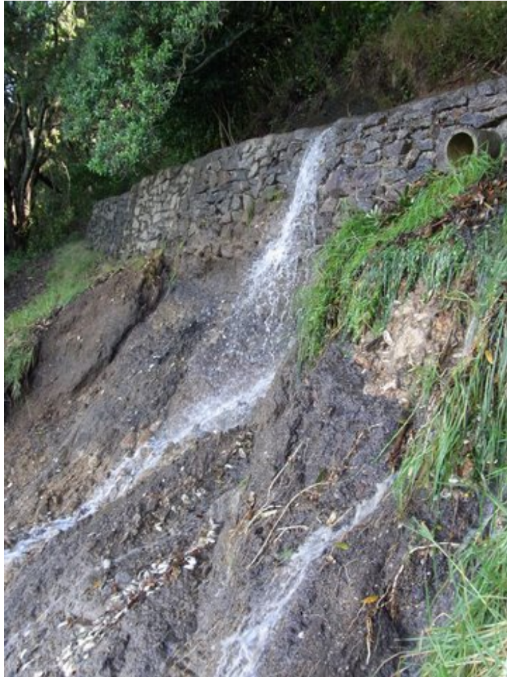
Scoured wall foundations
