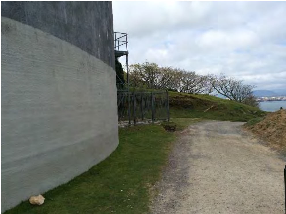
Figure 49: The water reservoir is subject to graffiti and vandalism on occasion. The current remedy is to paint over any graffiti at the first instance, this is not a more permanent and lasting solution. It is recommended to vegetate around the water reservoir to create a screen and barrier for anyone intending on vandalising it.
