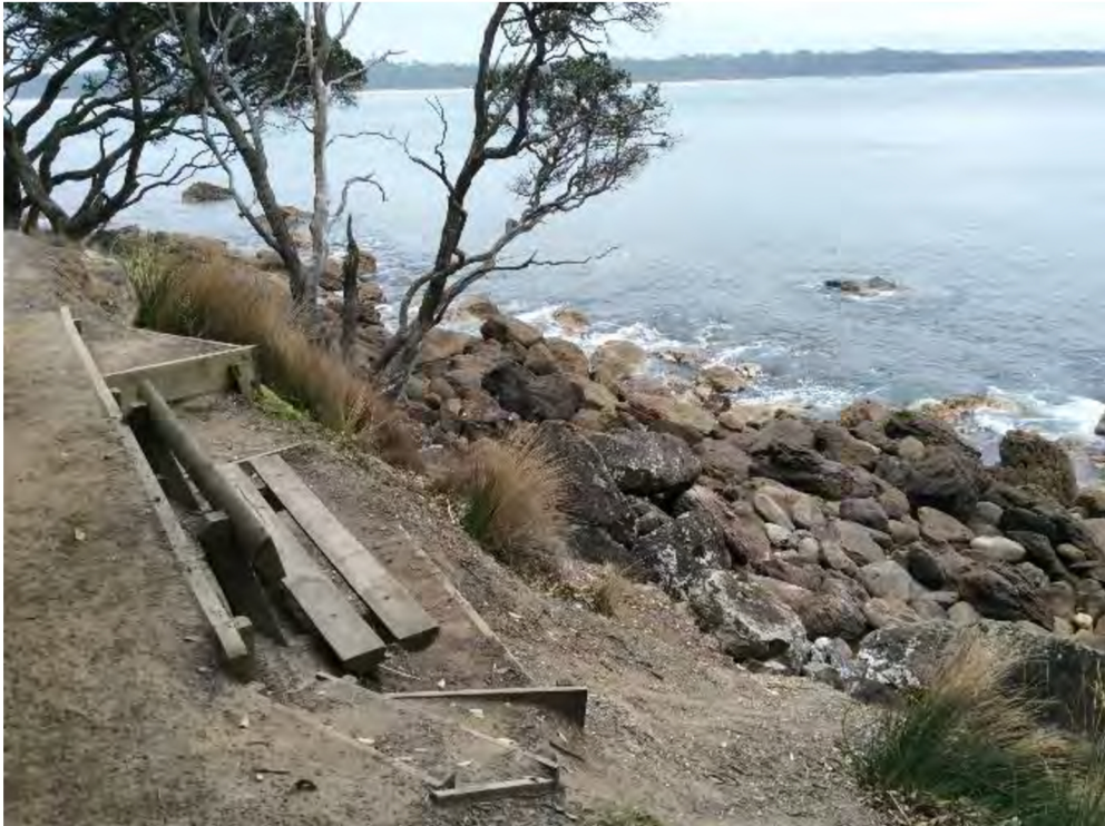
Figure 23: An older seat installed sunken down to track level looking over the western shore of Mauao. Seats of this age are to be removed in the near future and replaced with more modern seats.
