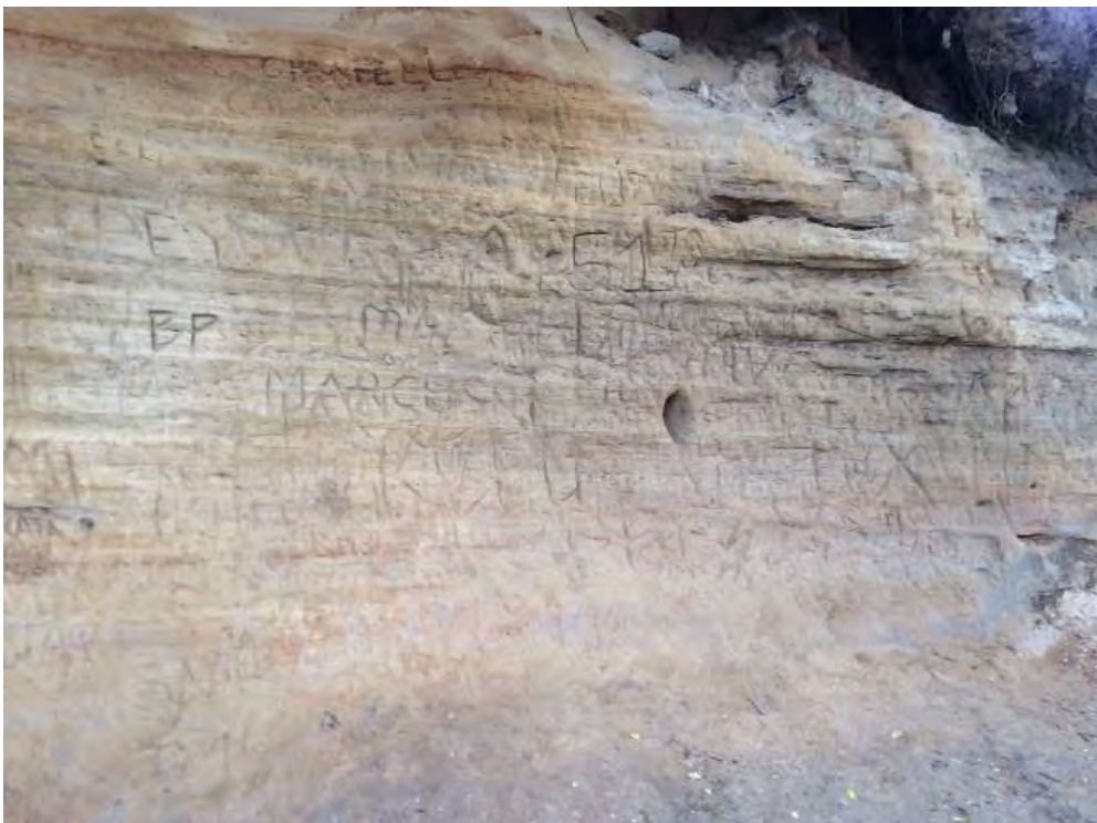
Figure 6: Exposed clay cliff faces to the inside of the track are subject to intentional gouging, particularly to chisel names into the clay. Over time this recedes the cliff face and causes instability. In one instance recently a costly stone retaining wall had to be installed to prevent collapse partly caused by this intentional gouging of the cliff face.
