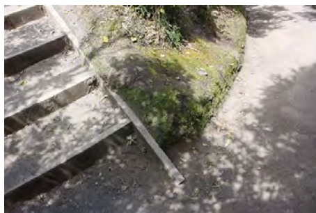
Figure 9 – Example of timber end of step protruding out into track corner
