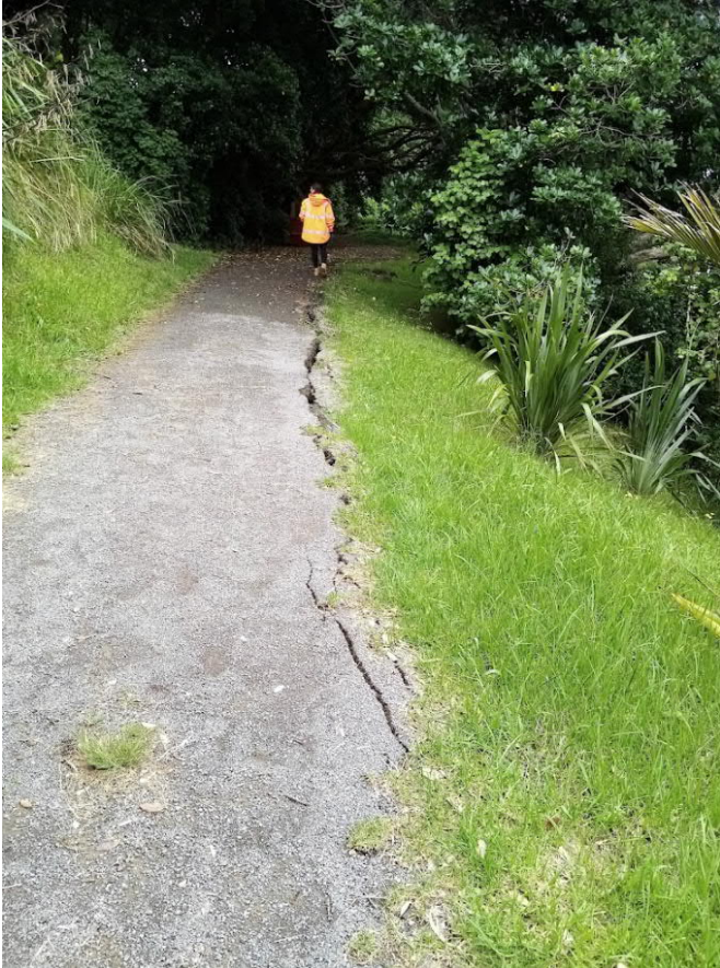
Figure 2: Tension crack along track
