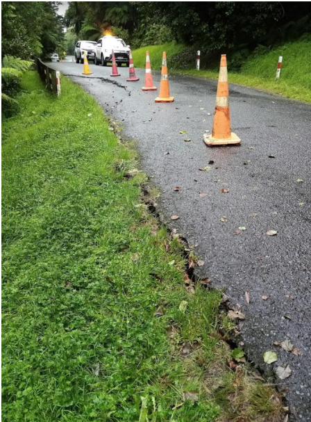
Figure 3: Straight section of tension crack.
