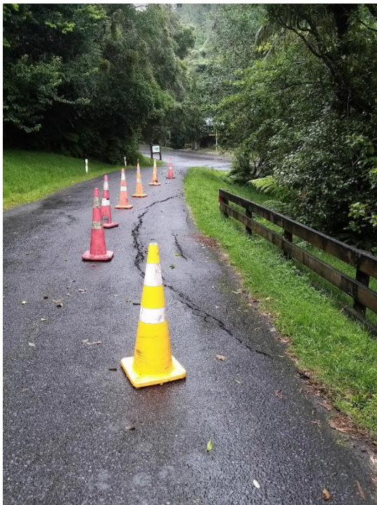
Figure 2: Arcuate section of slump and tension cracking in pavement
