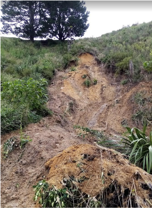
Figure 3: head scarp/ origin of failure
